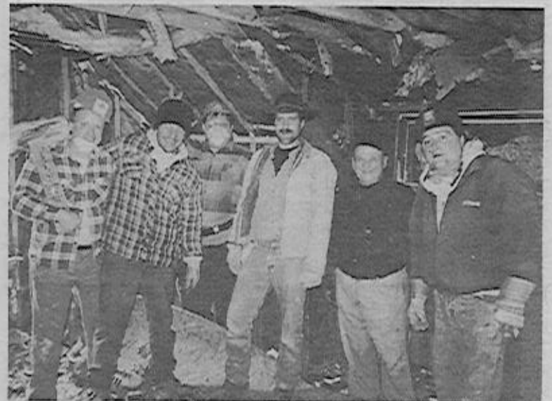
Larry Blazey, Carmen Valeri, Chuck Crevison, Gary Trescott, John Pascucci and Bart Bracaglia working in the attic of Number 10 Maple Street. (Photos by Don Tubman)
